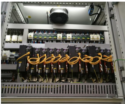
16 axis servo control system
